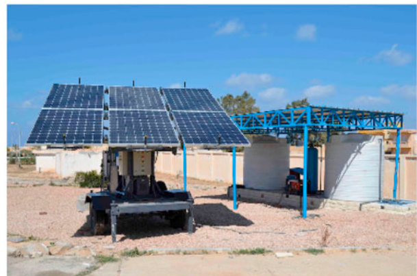
Fig. 7. Mobile PV/RO water desalination plant.
